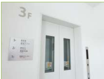
Elevator from 1 st floor to 3 rd floor
